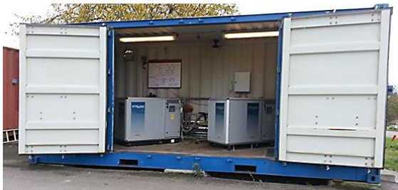
Figure 1. The two Stirling engines at Rönneholms waste management facility, [17].
