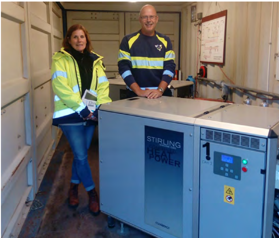
Figure 4. Maria Persson and Martin Svensson, MERAB, standing between the two Stirling engines at Rönneholms waste management facility, Sweden. Photo: Jörgen Held
